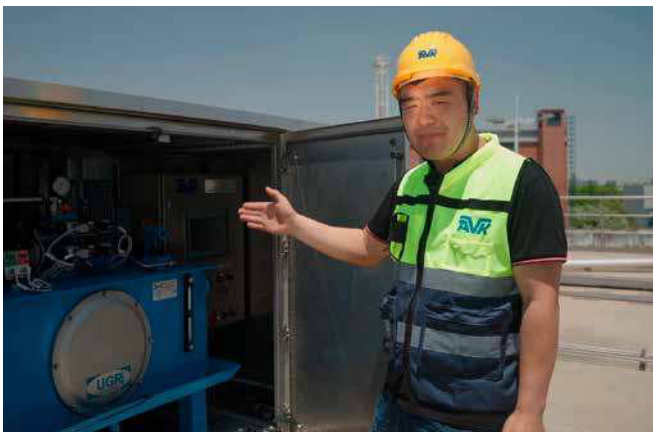
One of the weir penstock hydraulic control units finalised.
